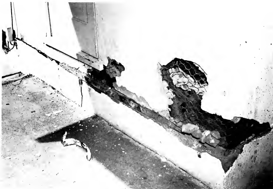
Photo 26. Motion between footings and exterior walls was often common in the areas of intense shaking.
